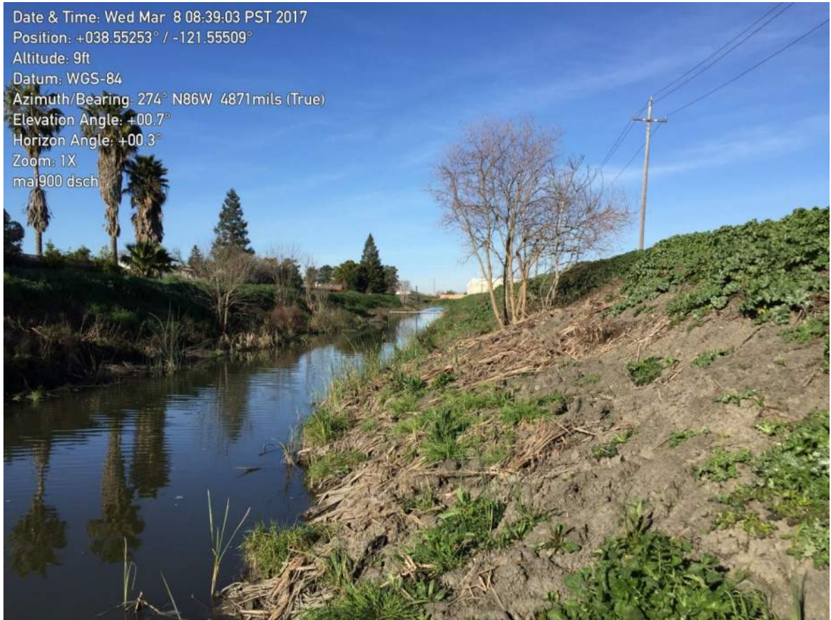
Photo 10-5 Main Drain Channel – Minor Bank Degradation
