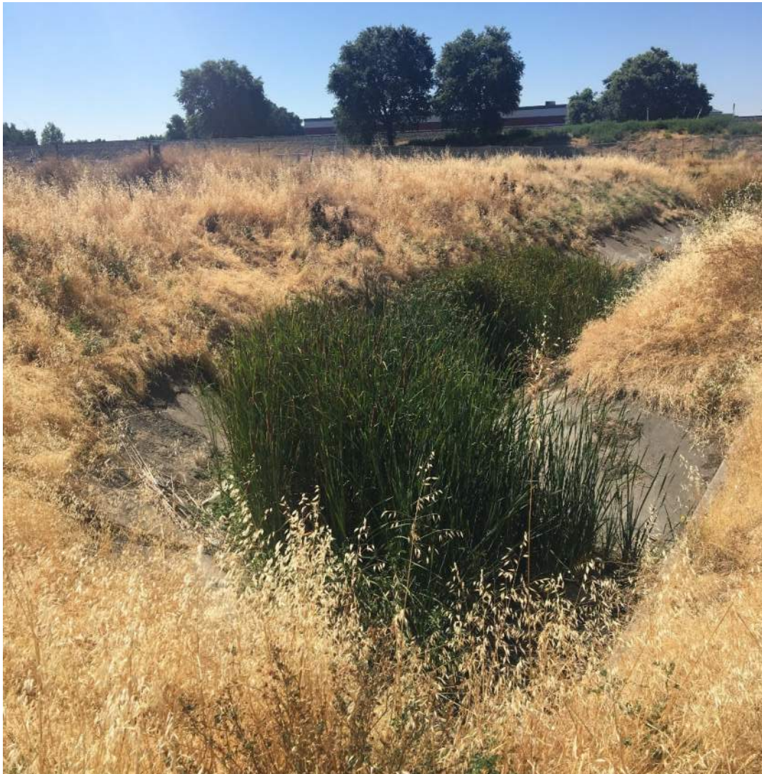
Photo 10-4 RD 537/RD 811 Channel – Heavy vegetation and mild sedimentation were observed upstream of Jefferson Boulevard
